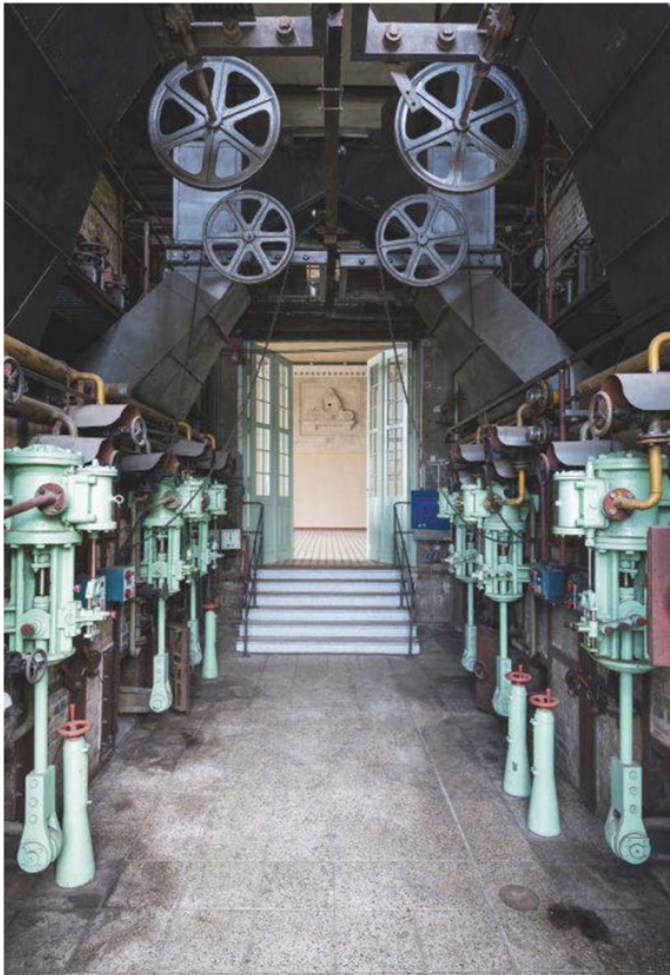
ABOVE, THE TURBINE HALL, WHICH WILL PLAY HOST TO A ROSTER OF PERFORMANCE ARTISTS AT THE POWER STATION'S OPENING LEFT, A LABYRINTH OF PIPES, FURNACES AND LADDERS IN THE ENGINE ROOM
